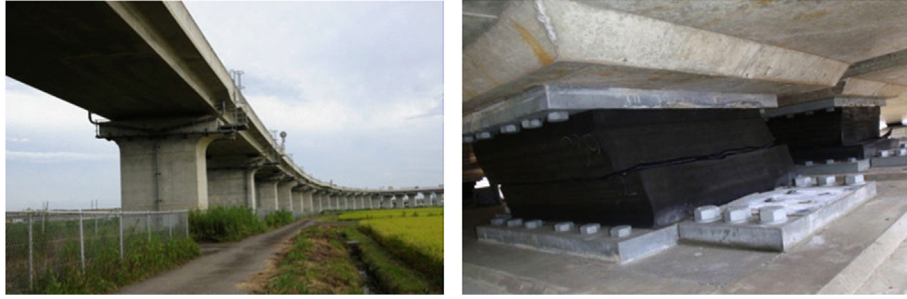
Fig. 5. Fracture of the bridge rubber bearing after the 2011 Great East Japan Earthquake (From Takahashi, 2012). Horizontal cracks are observed on the right.
